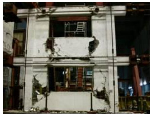
Photo 6. Specimen WWFER acted like a frame after wall failed
