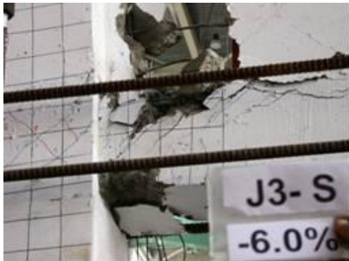
Photo 3. Beam end cracked after wall failed
