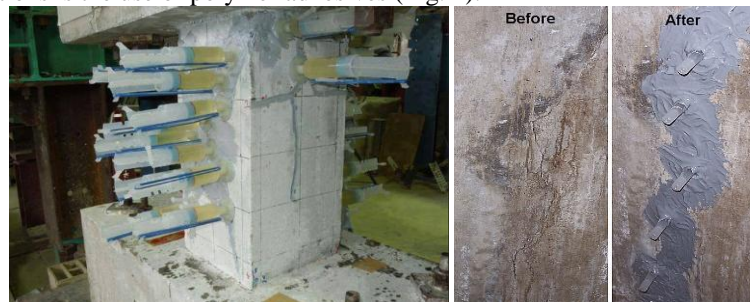
Fig. 2. Repair of cracks of concrete and reinforced concrete elements by polymer adhesive
