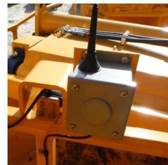
Fig 3 Wireless antenna on top of machine
