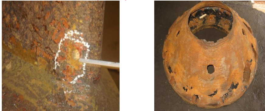
Fig 12: Corroded/Eroded Hydro-mechanical Components
