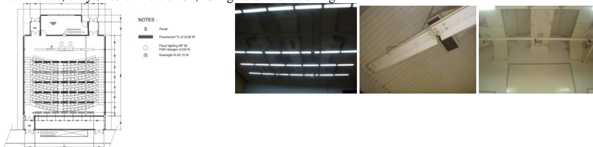
Fig. 3. Lighting installation of lecture theatre (source: survey documentations, 2008)
